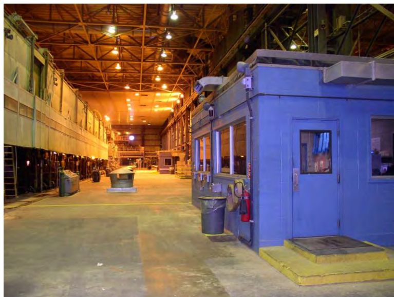
Figure 4.30 - Acoustical control room and noise refuge in a paper manufacturing facility
