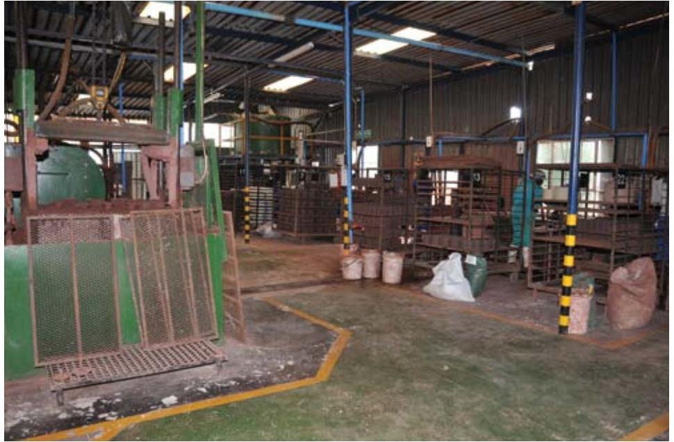
In the sleeve making plant considerable work was done. The ovens were refurbished, the floor was restored, the drainage was overhauled, the pressure vessel was replaced and piping was completely replaced
