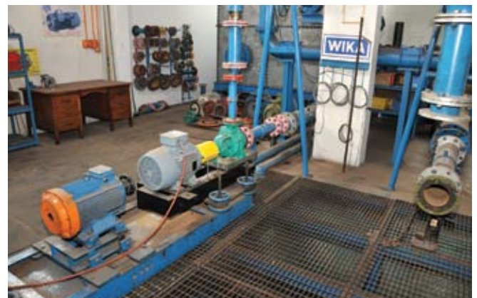
The company has a fully operational test-bed enabling it to carry out the testing of pumps at the factory
