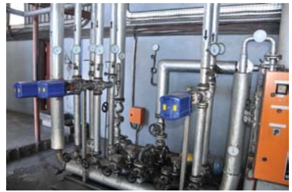
The new thermo-oil system
