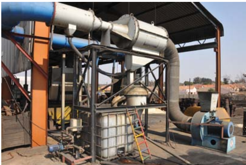
The company purchased a larger baghouse/dust extractor and a wet scrubber, approximately two years ago
