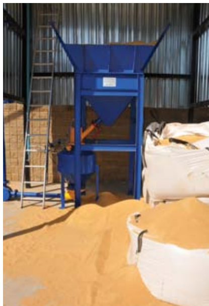
The Lauds sand delivery system, which includes a fully automated 5TPH pneumatic conveyor with all the necessary controls for the five ton dry silica sand hopper. The hopper feeds the two Lauds mixers and has a vent unit attached to ensure no dust is present during operations of the filling cycles
