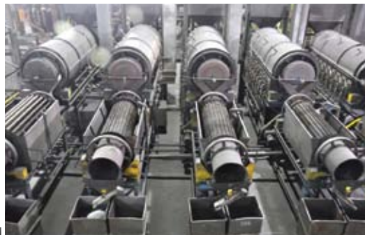
Four new LNG gas fired tempering furnaces, each with water quench, were installed
