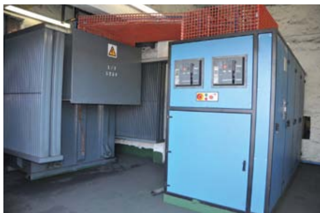
The new Solid State 1.5 megawatt medium frequency furnace was installed earlier this year
