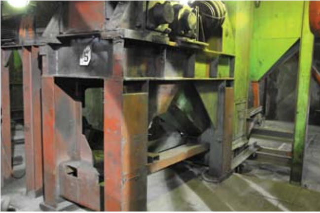
Crushing capacity was increased by 40% with the installation of four further crushers, built in South Africa but based on group design
